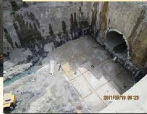
Esfahan Kargar Metro Station
